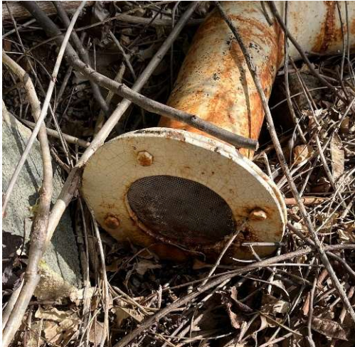
Falls Avenue tank overflow before installation of flapper valve
